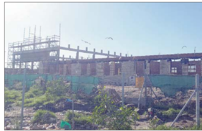
GOING UP: New buildings are under construction and are expected to be finished in December. The 1 500 pupils are currently housed in 38 temporary structures.
